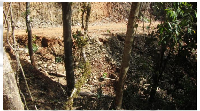
Photo-8: Unstable road fill material without retaining wall near Sasiguli.
