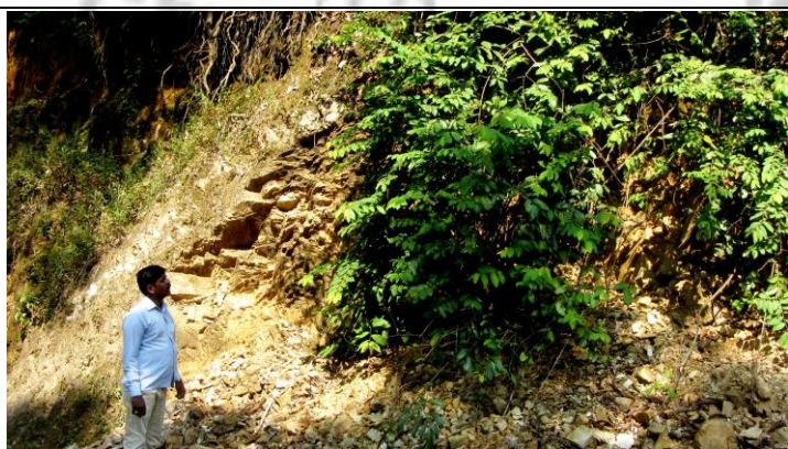
Photo-3: Wedge failure in Argillite, slide no. KAR/UK/48J11/2014/02.
