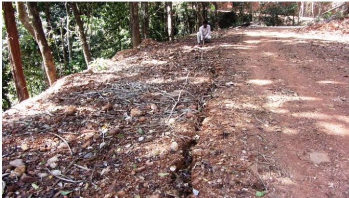
Photo-7: Development of cracks in road fill material near Sasiguli.
