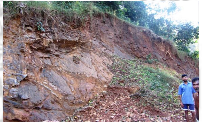
Photo-10: Planar wedge failure in schist near Sasiguli, KAR/UK/48J11/2014/16.
