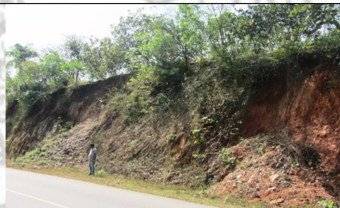
Photo-4: Slide due to extensive road cutting, slide no. KAR/UK/48J11/2014/07.
